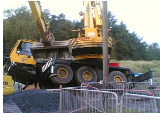
Picture of a crane that Nearly overturned on a MJ Gleeson site
